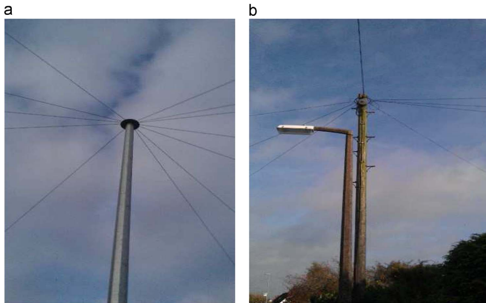
Fig. 1. (a) Existing landline end user connectivity (UK) and (b) Co-existence of both landline and streetlight infrastructure (UK).
