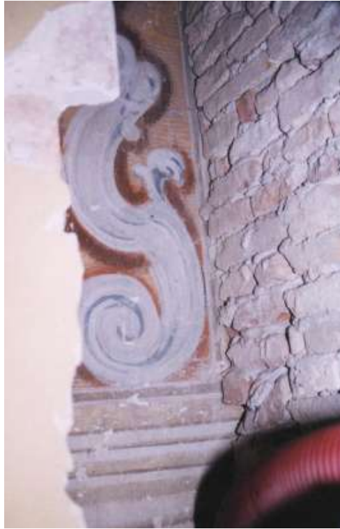
Fig 8: Excavated semicircular niche of 1852-5, set into fifteenth-century arched recess (west wall), showing frescoed designs of c1718. Photo: authors.
