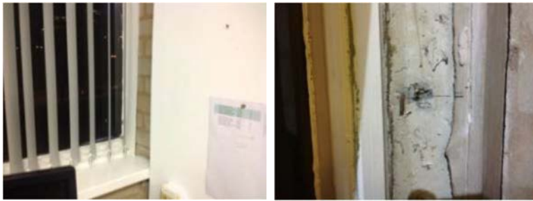
Figure 4: Detail of the loose insulation containing asbestos around screw holes found.
