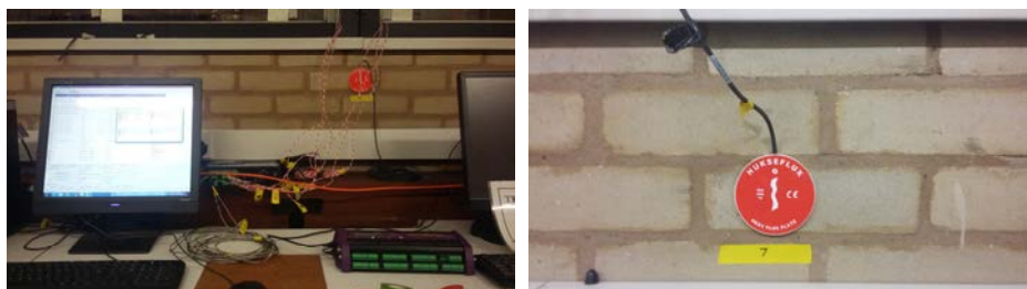
Figure 8: Non-invasive monitoring equipment installed.
