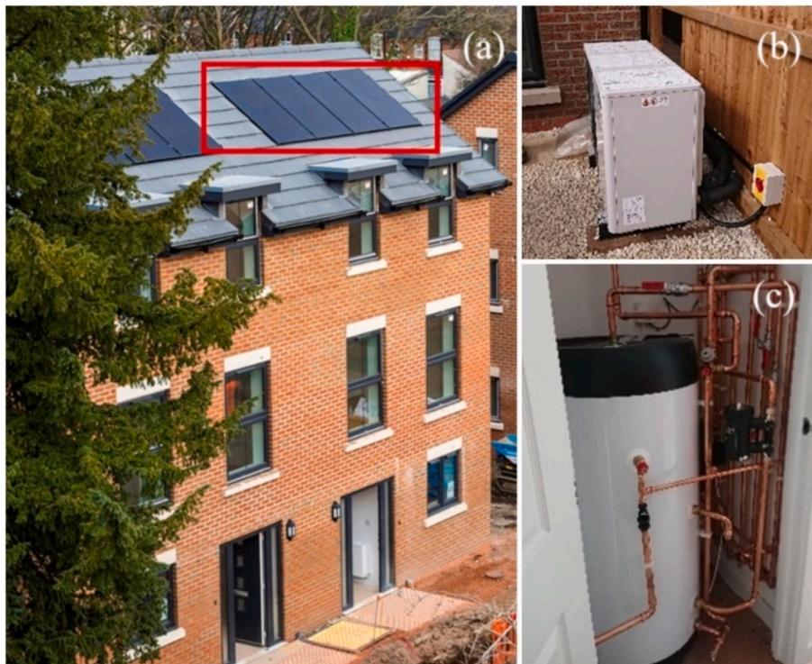
Fig. 2. Photographs of installed (a) solar PV array, (b) heat pumps and (c) hot water cylinders.
