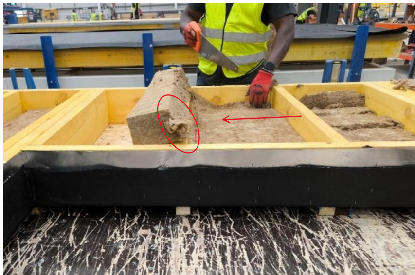
Figure 5.23: Rockwool insulation overstuffing practice
