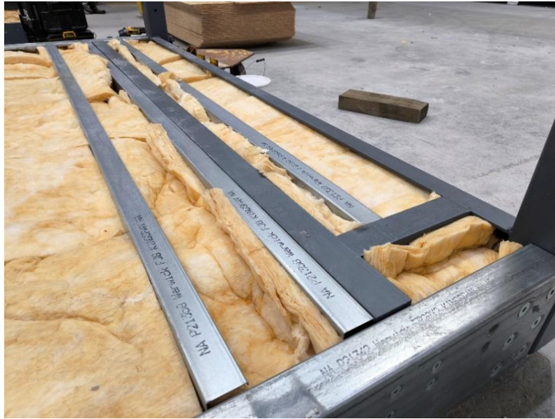
Figure 5.10: Rockwool insulation overstuffing practice
